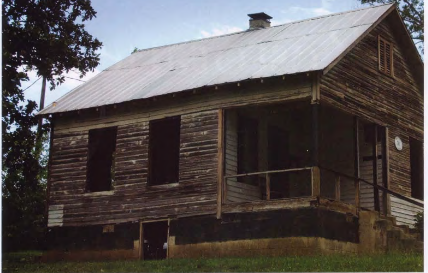
The modest frame building on East Livingston Street in Tryon is being restored. Eunice Waymon, known to the world as the legendary musician Nina Simone, was born in Tryon in 1933.
